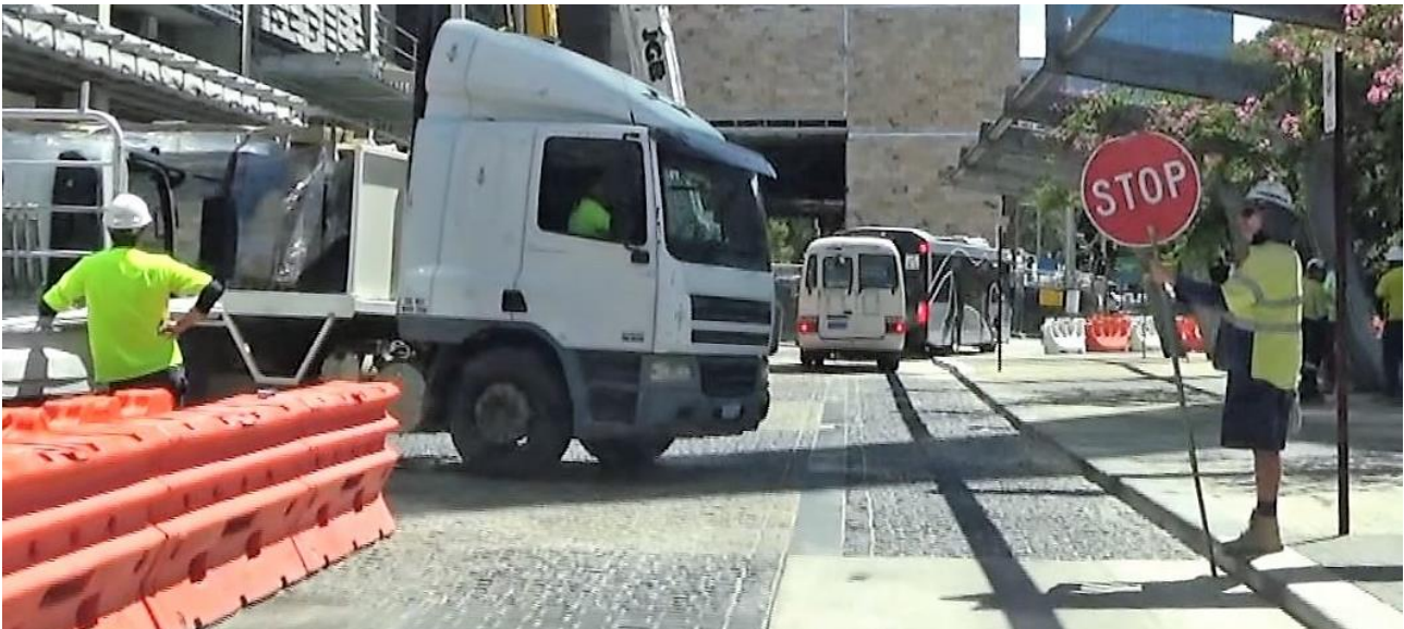
Example of faded hi-vis clothing on traffic controller on right compared to new hi-vis on left
